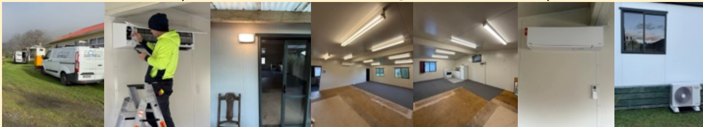
Daryn – New LED lights & heat pump installed 21 July [4Regions+NZCT+DIA+NHC]
